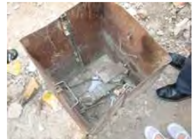
9. Backflow valve in access shaft.
