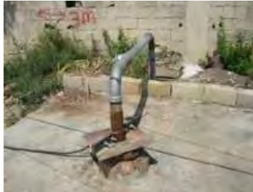
14. Well head (water source for entire camp). This is where the proposed emergency power generator and sound-proof room will be located.
